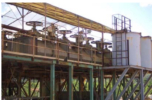
Redbank flotation plant for treatment of sulphides (to be refurbished)
